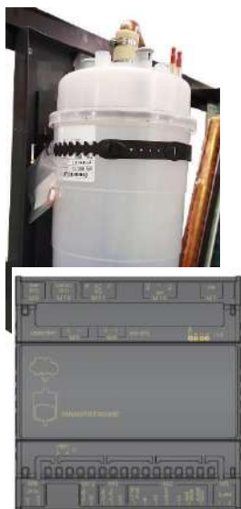
Humidifier control board
